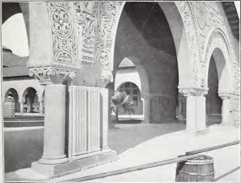
B. EARTHQUAKE EFFECT ON ARCHES, LELAND STANFORD JUNIOR UNIVERSITY.
